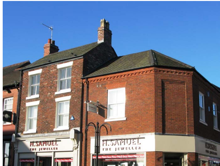
Here at the corner of Castle Walks, something close to imitation was the best solution. (The building on the right hand side is about 200 years younger than its neighbour.) © SueC
